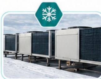
REFRIGERATION & AIR CONDITIONING
